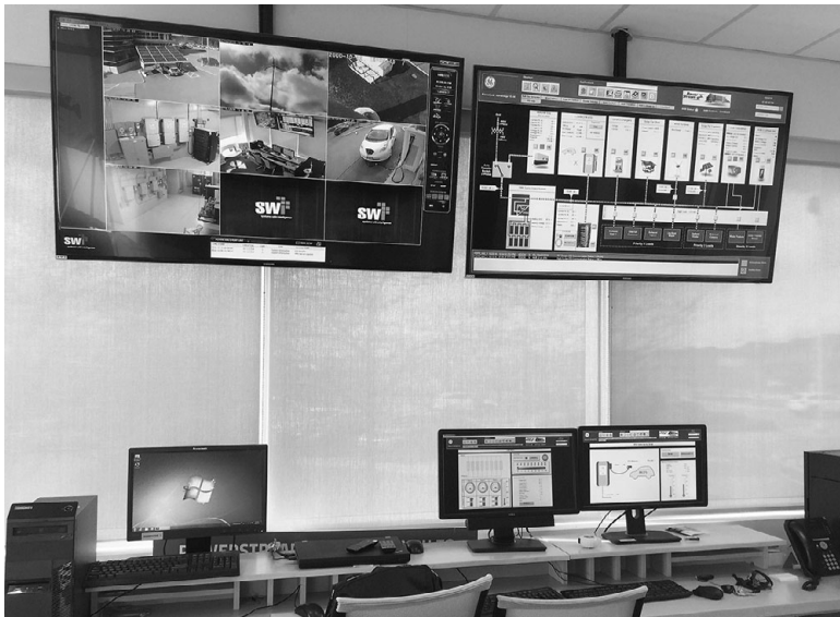
Figure 2.2 A microgrid control room at Alectra Utilities (formerly PowerStream).
