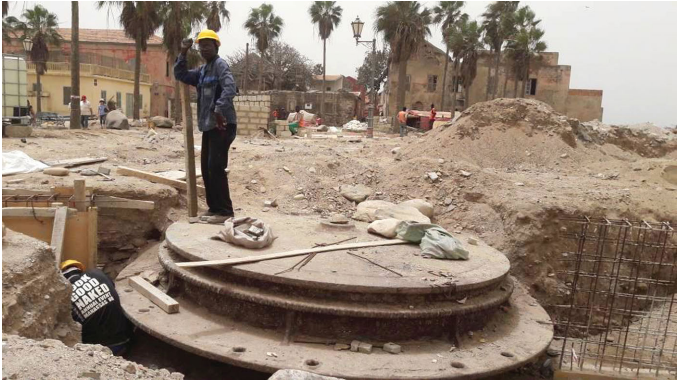
FIGURE 3. Construction works occurring on Gorée Island without any archaeological involvement (Photograph, I. Thiaw).
