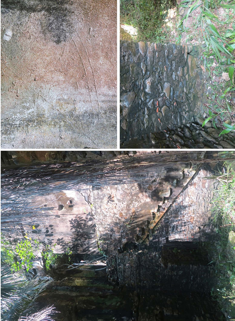
Figure 5. Access to upper floor and graffiti. Lower level shows evidence of scorching (photograph by M.D. Cruz).
