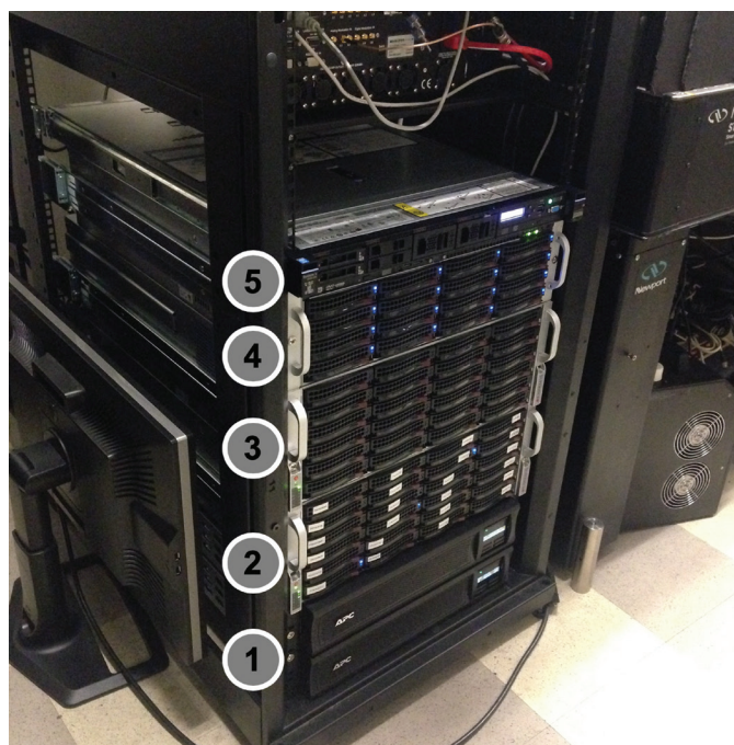
Figure 3: Organization of servers. From the bottom up: (1) Two redundant UPS units, (2) main storage server, (3) JBOD expansion, (4) analysis computer, (5) web server for https://fliptrap.org . All servers are mounted in a standardized 19-inch-wide server rack using supplied rails.
