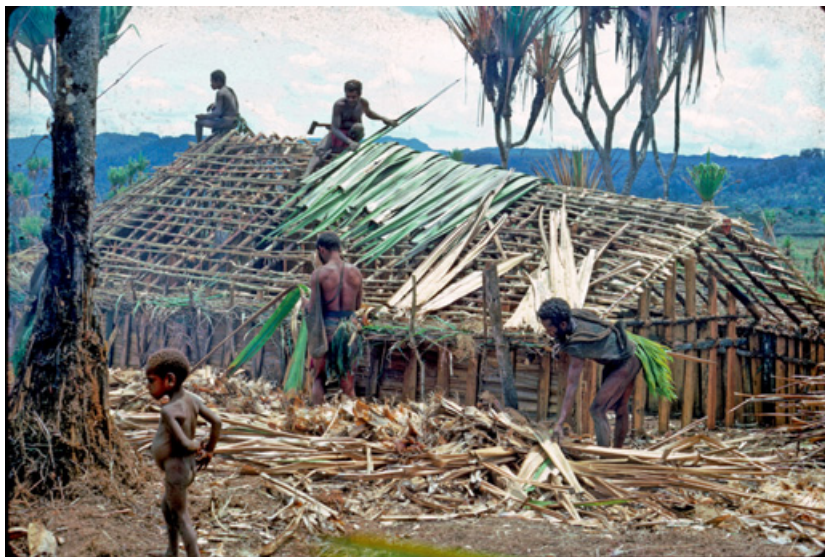
Figure 3 Men building a traditional house (courtesy of Paul and Ruth Wohlt, Yumbisa, northern Kandep, 1973)
