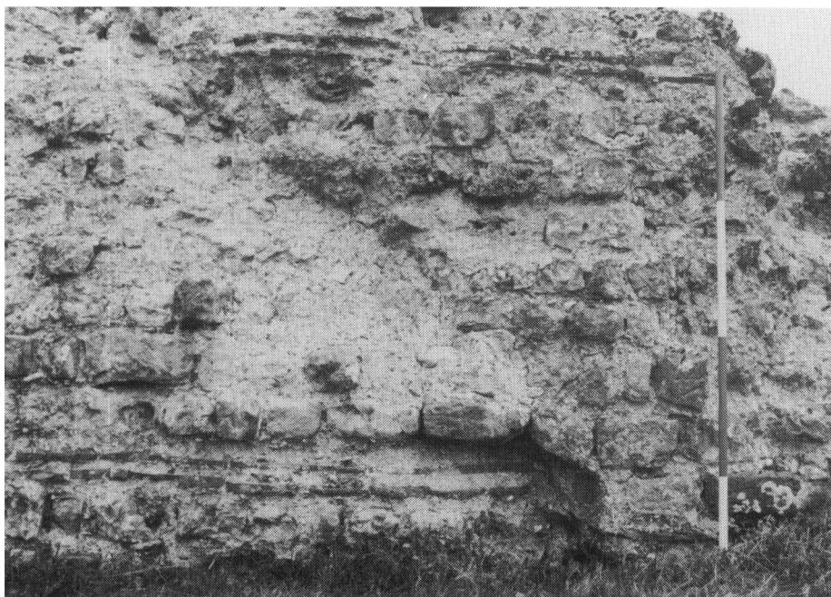
B. Lypne. The north wall of the fort showing the join between two working-parties (p. 232).
