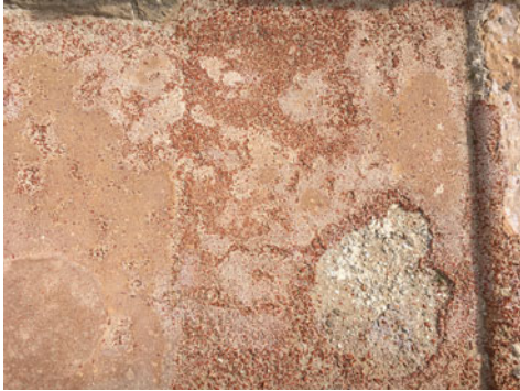
Figure 1. Roman opus signinum from a domestic cistern in Lucentum (Alicante, Spain). Note the remains of the smooth surface (left); smoothing closes the pores, thus improving impermeabilization. Here, the lining was applied on top of a base layer of sand-lime mortar.
