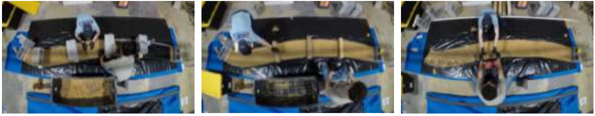
Figure 6. In step 2, the formwork is packed with living myco-materials. Photos by Jonathan
