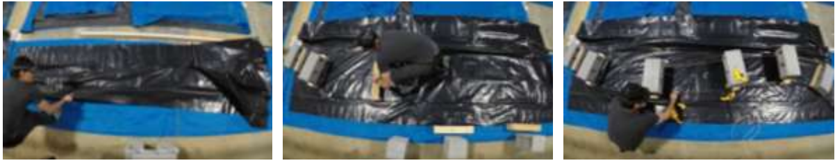
Figure 5. In step 1, formwork is laid out on an impermeable membrane. Photos by Jonathan
