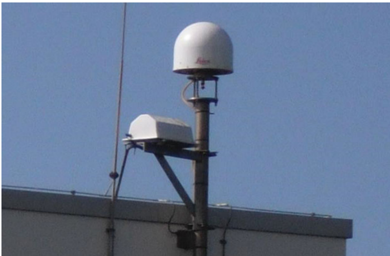
Fig. 20. GNSS station at IJmuiden, the Netherlands, with a co-located active radar transponder. Hereby, GNSS measurements and PSI measurements can be connected in the same geodetic datum. The GNSS receiver is placed within the round dome, whereas the radar transponder is contained within the white box.
