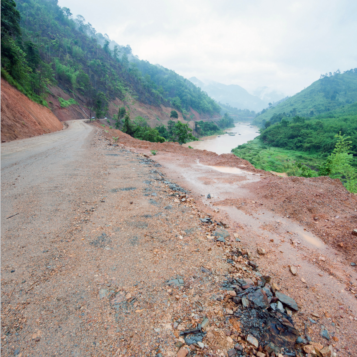
Photo: The Dawei road link currently remains unpaved, and already the majority of adjacent slopes have been deforested. The project's scope has varied greatly over time, alternating between eight-, four-, and two-lane alignments, with and without rail, power lines and gas pipelines. © Atid Kiattisaksiri/LightRocket via Getty Images.
