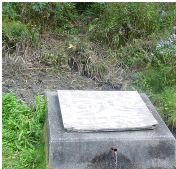
Fig. 1. Roadside spring box on 17 September 2009, located on Route 22 in the town of Stephentown, Rensselaer County, New York.
