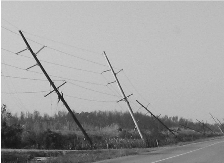
Figure 2.24 Overhead transmission line using both wooden (darker colored) and metallic (lighter colored) poles. This line was damaged by Hurricane Ike.
