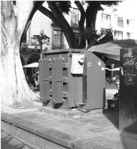
Figure 2.41 A pad-mounted transformer.
