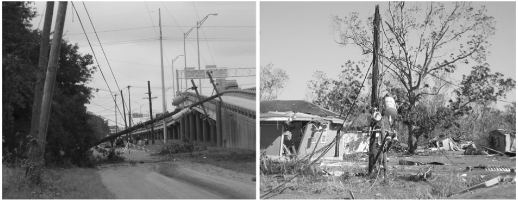
Figure 2.48 Transformers damaged due to strong winds.
