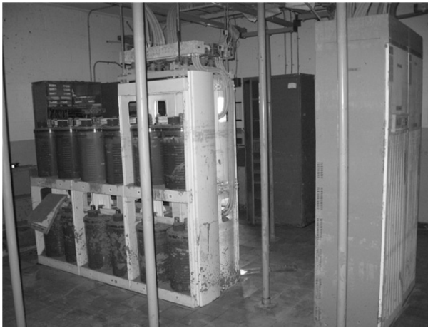
Figure 2.63 Rectifier cabinets (right) and batteries (left) in a CO flooded by Hurricane Katrina.
