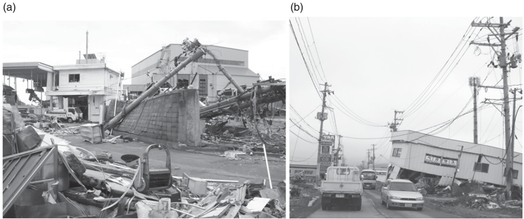
Figure 2.47 Pole-mounted transformers after an earthquake and tsunami. (a) Transformer damaged due to a fallen pole. (b) Undamaged transformers.
