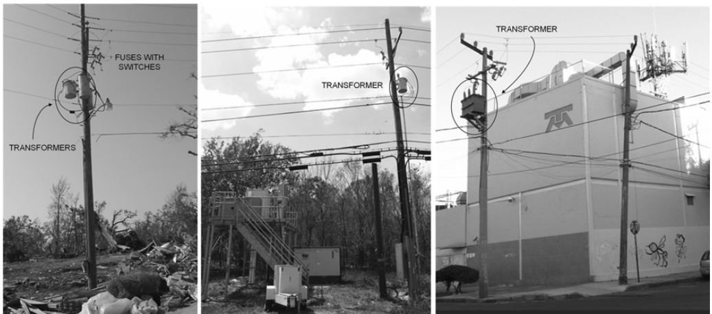
Figure 2.40 Examples of pole-mounted transformers.
