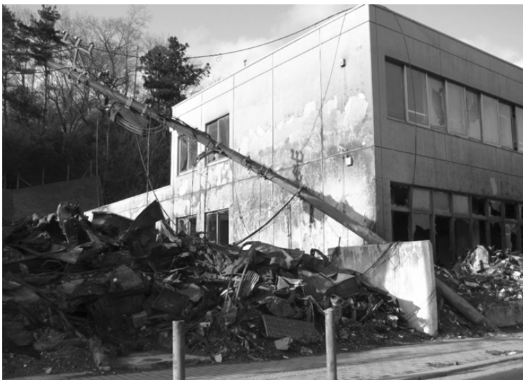
Figure 2.93 Fire damage caused by burning debris carried by tsunami waves.
