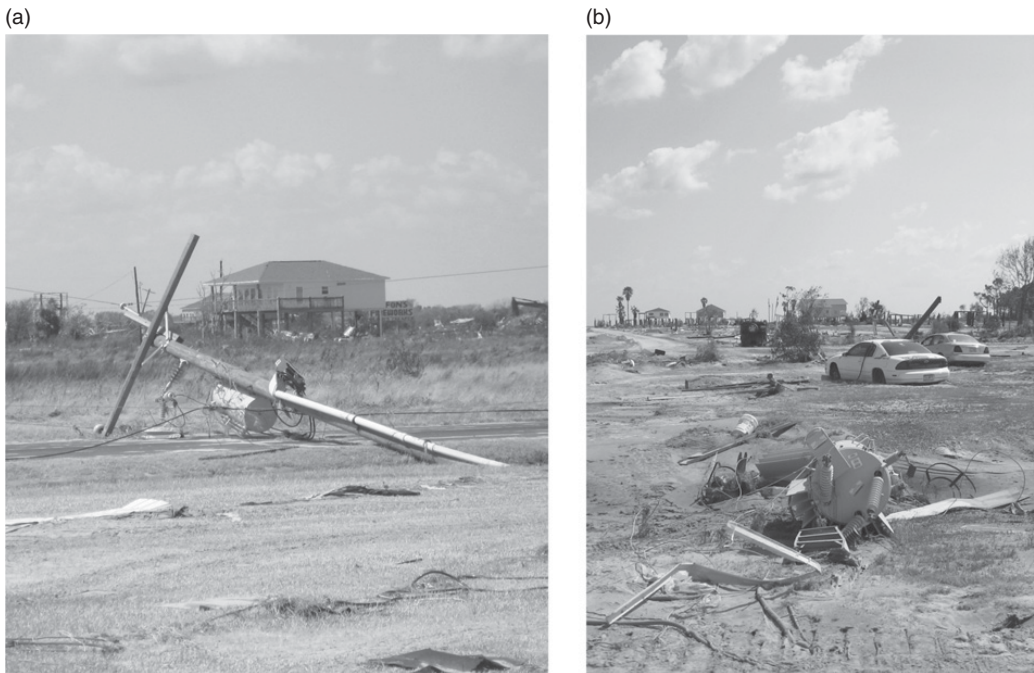
Figure 2.46 Damaged transformers after a hurricane. The one shown in (a) was damaged by pole failure.
