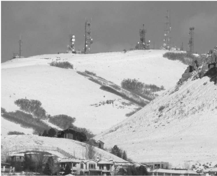
Figure 2.66 Microwave radio repeaters on top of a mountain.
