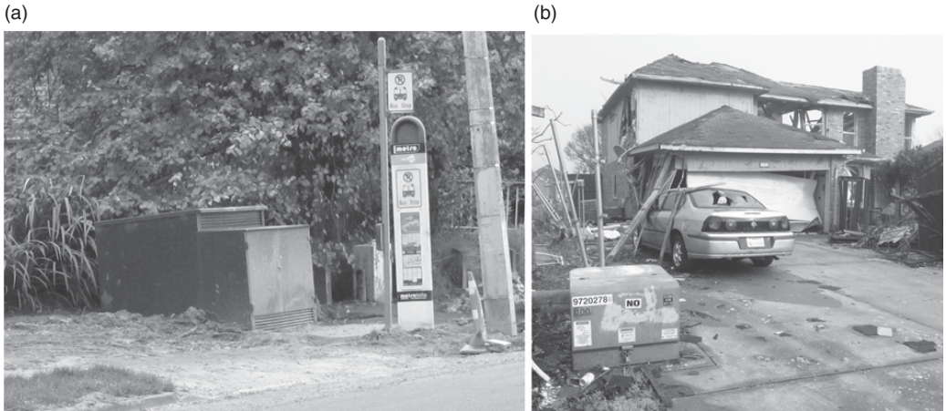
Figure 2.43 Pad-mounted transformers after natural disasters. (a) After an earthquake. (b) After a tornado.
