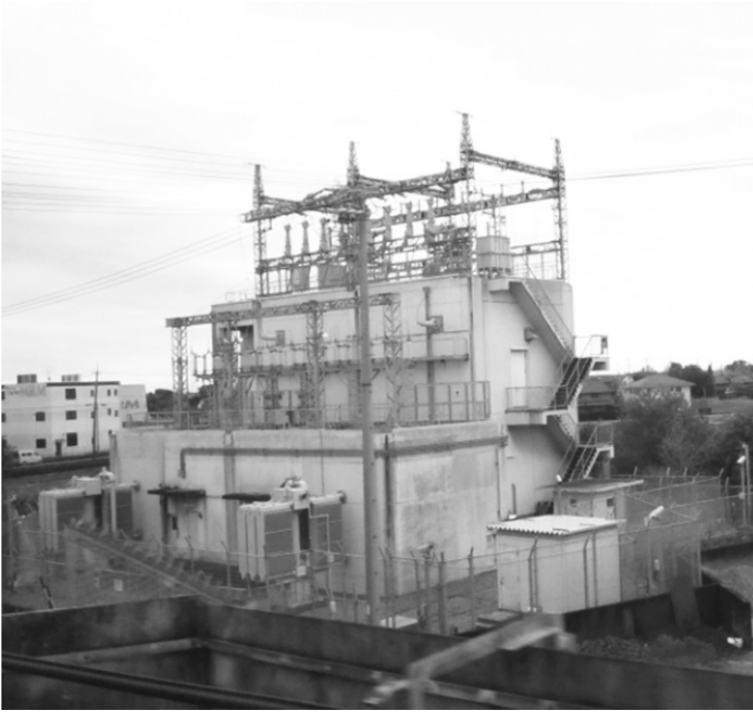
Figure 2.36 Example of a compact aboveground substation in an urban area in Japan.
