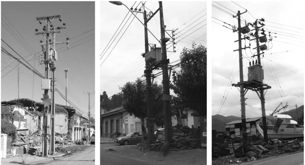
Figure 2.44 Overhead transformers on platforms after earthquakes and tsunamis.
