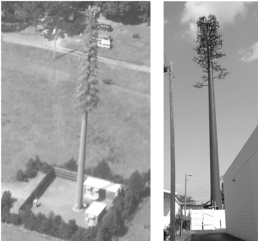
Figure 2.77 Examples of cellular towers disguised as trees.
