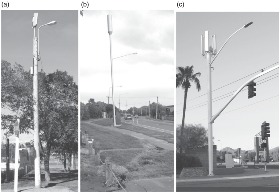
Figure 2.81 Examples of small cell sites mounted on streetlight poles. The earth crack shown in (b) was caused by an earthquake.
