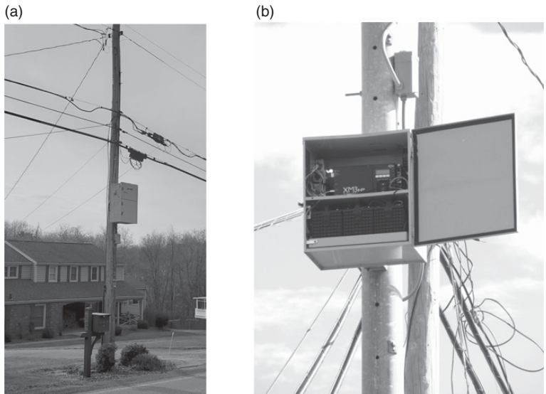
Figure 2.60 (a) A CATV UPS mounted on a pole and (b) a similar CATV UPS also mounted on a pole with its door open, showing the batteries on the bottom shelf.
