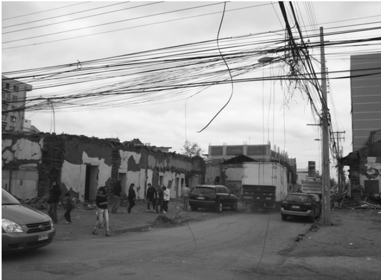
Figure 2.51 Example of a power distribution circuit with a dense run of conductors (some of them could also be telephony cables).
