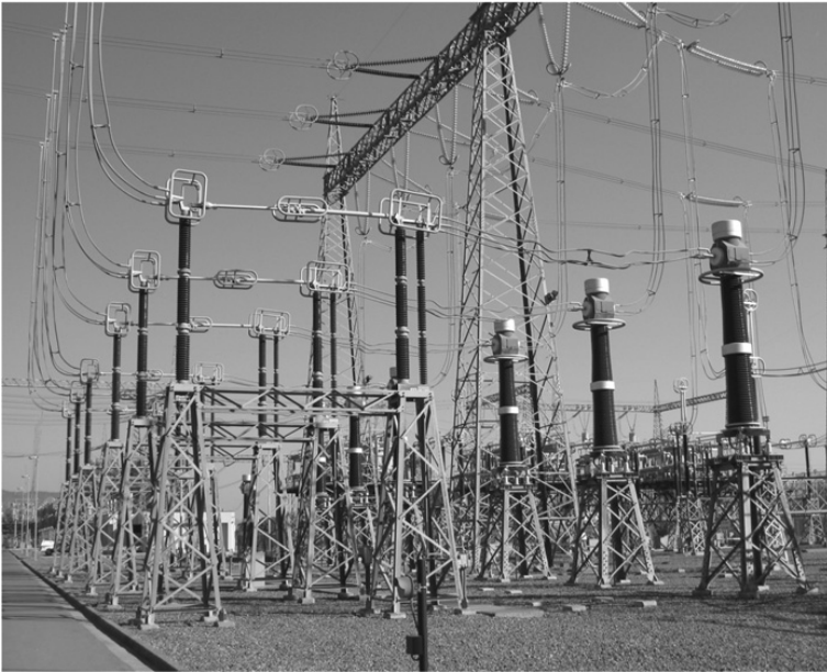
Figure 2.30 Horizontal semi-pantograph (on the left) connected to current transformers (on the right).
