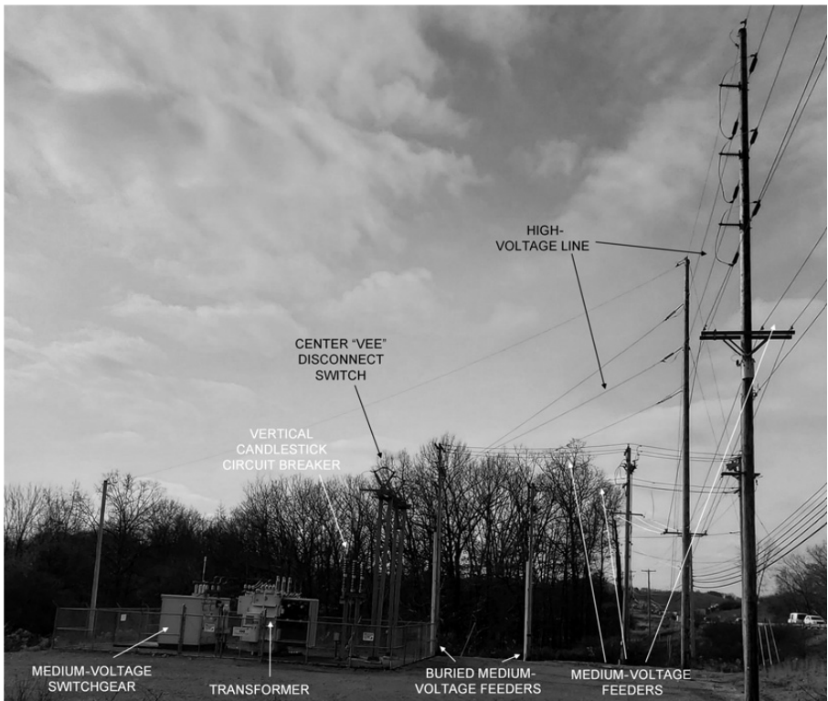
Figure 2.38 A typical distribution substation in the United States.
