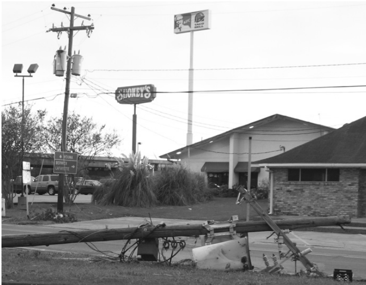
Figure 2.50 A fallen pole with transformers causing loss of power to consumers connected to this transformer. Notice that electric power service is on across the street.
