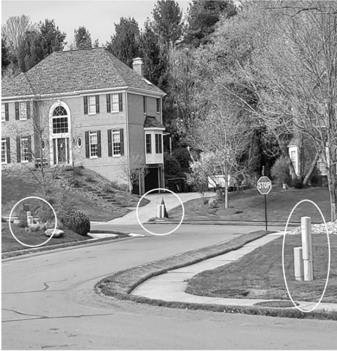
Figure 2.69 Underground telephone outside plant network with tap enclosures and connectors marked with circles.
