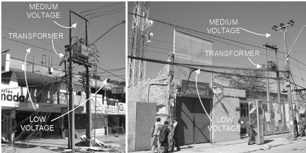
Figure 2.42 Overhead transformers mounted on platforms.
