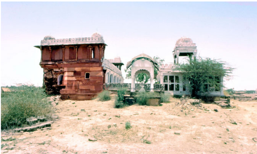
Figure 5. (Colour online) Mosque and tomb of Bībī Zarrīna, southern façade. The severely dilapidated rear wall of the mosque can be seen on the left. The tomb in the foreground with a “Bengali” roof dates from the late or post-Mughal era.
