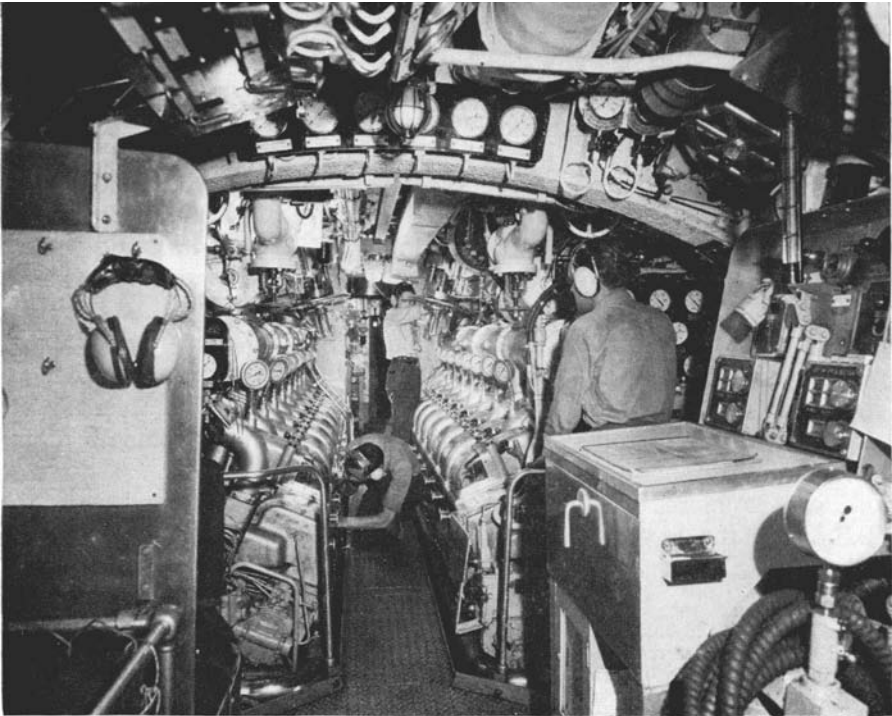
(b) Diesel engines (official Navy photograph).
