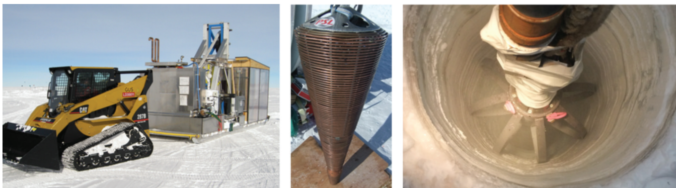
Fig. 5. (Left) independent firm drill sled; (middle) independent firm drill copper coiled cone; (right) IceCube drill head descending into a firm hole drilled by the independent firm drill.
