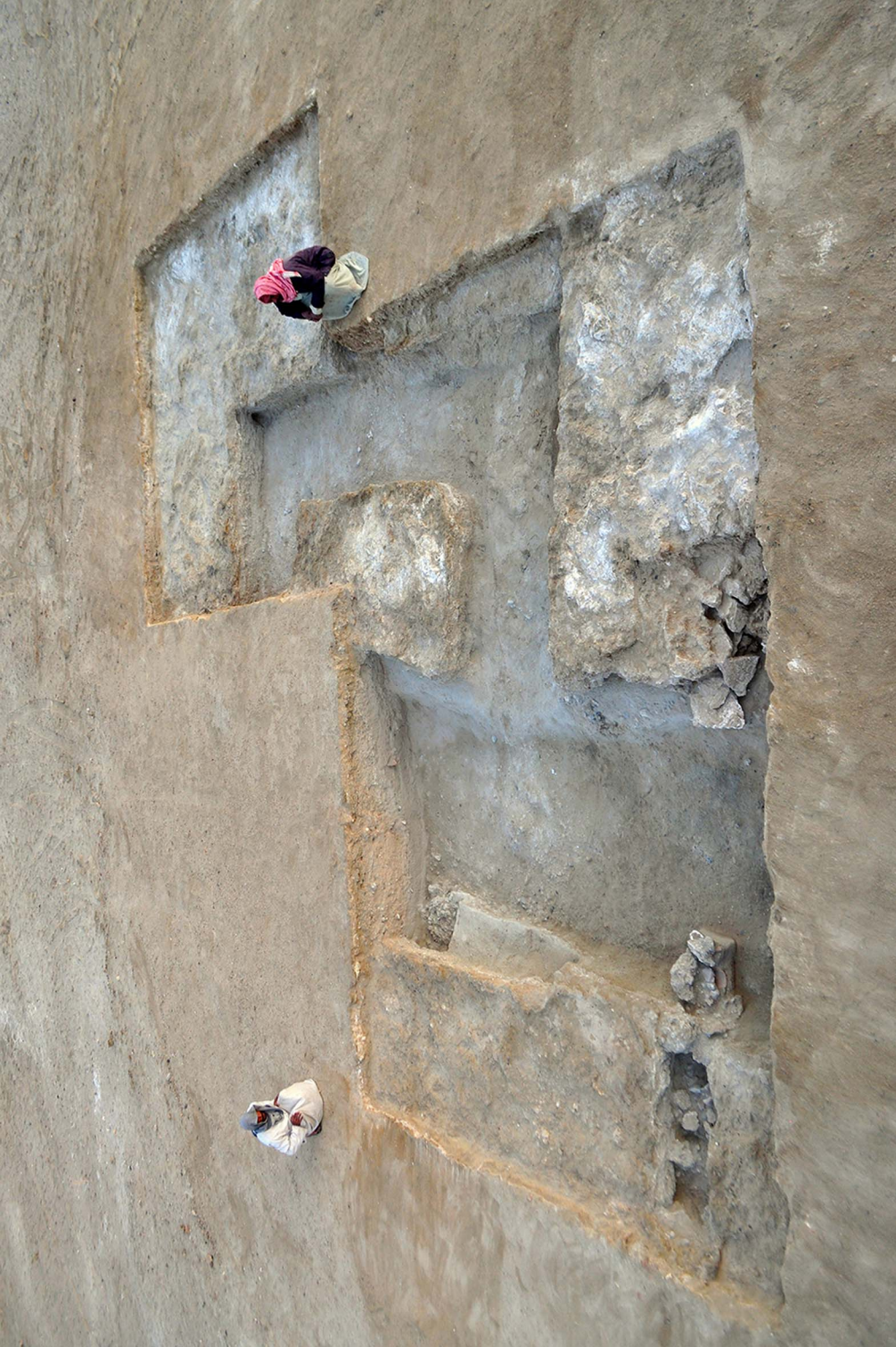
Figure 1. Complex of rock-cut foundation trenches of the north-western tower of a defensive/industrial building, viewed from the south (photograph by S.E. Sideboham).
