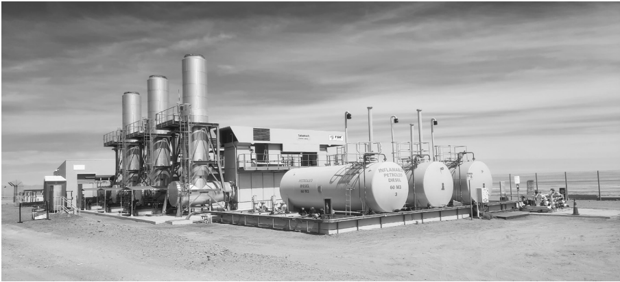
Figure 9.2 The ALMA power plant built by TSK Elektronika y Electricidad S.A. The plant uses Taurus 60 gas turbine generators, by Solar Turbines. The three 60,000 L fuel tanks on the right side of the photograph store diesel fuel; an additional three tanks, not visible, store 200,000 L each of LPG, enough to run ALMA for three days. Credit: ALMA/ESO/AUI/NINS, CC BY 4.0.
