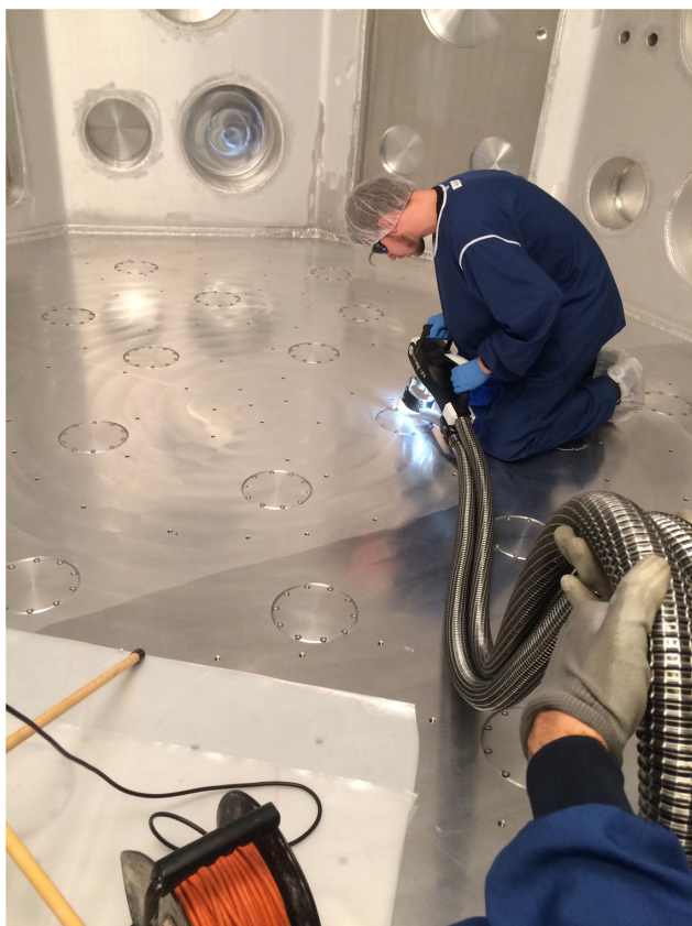
Figure 19. Cleaning of the P3 chamber floor shows a clear visual difference between the cleaned surface area and the non-cleaned area [31] .
