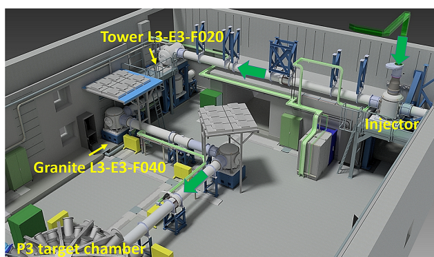
Figure 4. 3D CAD visualization of the HAPLS BT from the injector chamber to the P3 chamber. This figure shows the actual installation in E3.
