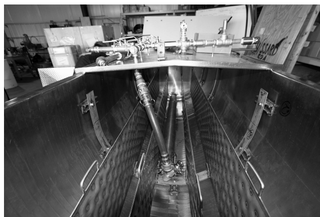
Fig. 3. The melt tank interior during build showing heat exchange plates and submersible transfer pump lying in the bottom of the tank. The manifold system can be seen in profile atop the tank.
