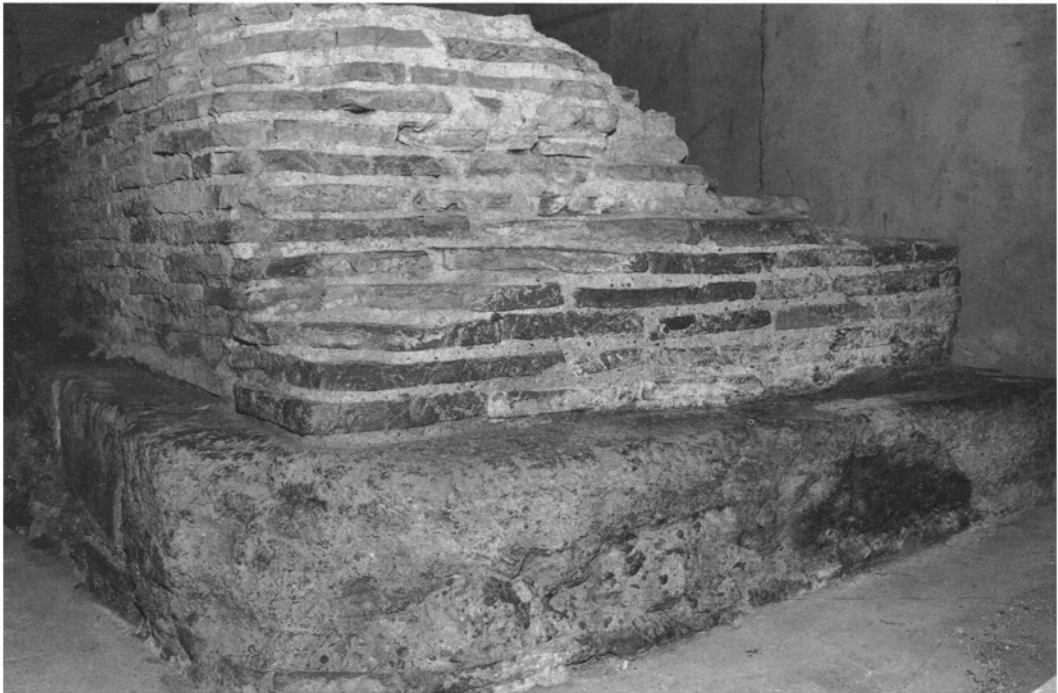
B. London Basilica: pier in Nave. Tile pier built over stone plinth dividing Nave from S Aisle in second- and third-century Basilica: cf. PL. XIII A. Pier recorded in 1881, and still survives in basement of 90 Gracechurch Street, standing 0.7 m high. (p. 68)
