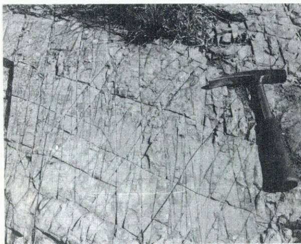
Fig. 5. Three joint sets on a pavement of light grey claystone; Khalaqah district.
