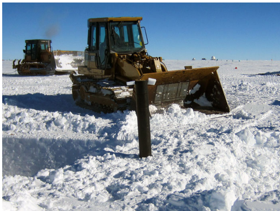
Fig. 10. At the conclusion of the project, the drill trench, drill slot and core storage trench were backfilled with snow. The borehole casing (image center) was extended ~1.22 m (4 ft) above the snow surface and the drill fluid was left in the borehole to facilitate future borehole logging or sampling.
