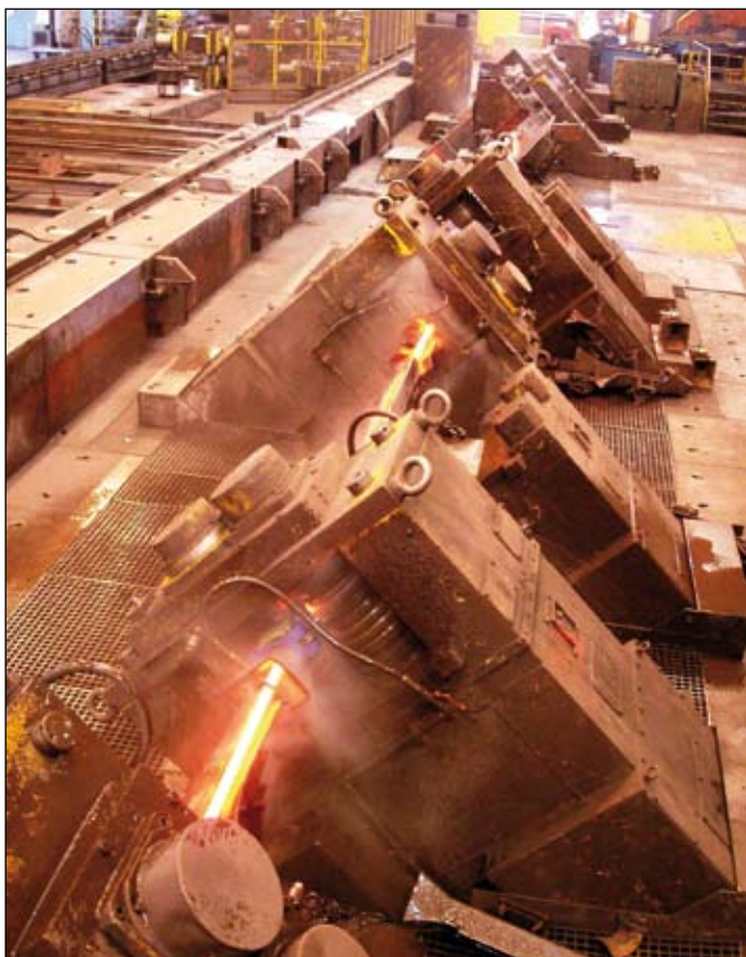
New drive and automation equipment on the continuous rolling mill, which has been in operation since 1988. Photo courtesy of Siemens
