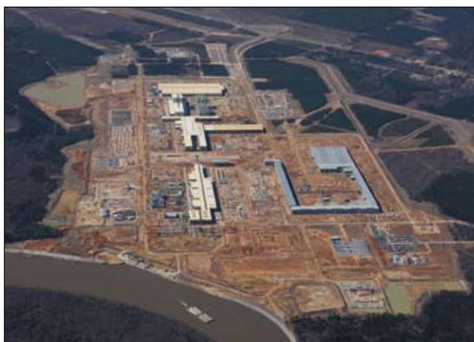
Since 2007 ThyssenKrupp Steel USA and ThyssenKrupp Stainless USA have been working together for the erection of the new plant for steel and stainless steel flat products in Alabama.
