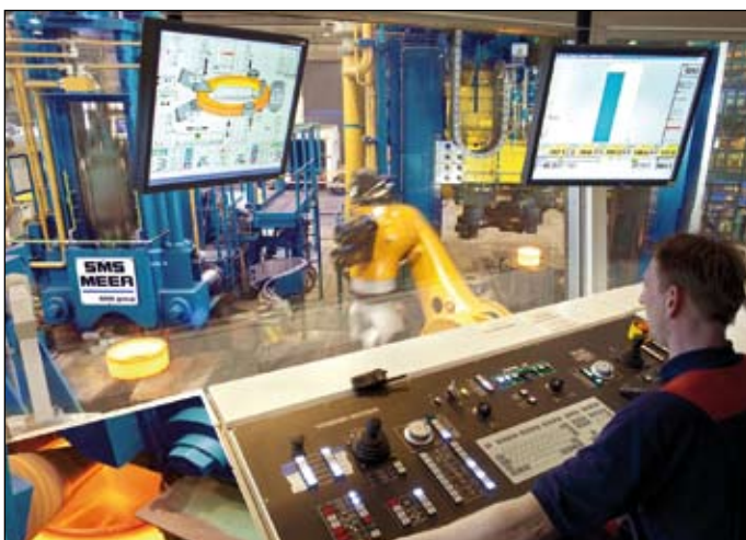
The new RiWa 2000/80 ring rolling plant must increase the annual capacity of the Ovako works to 55,000 t. Photo courtesy of SMS Meer
