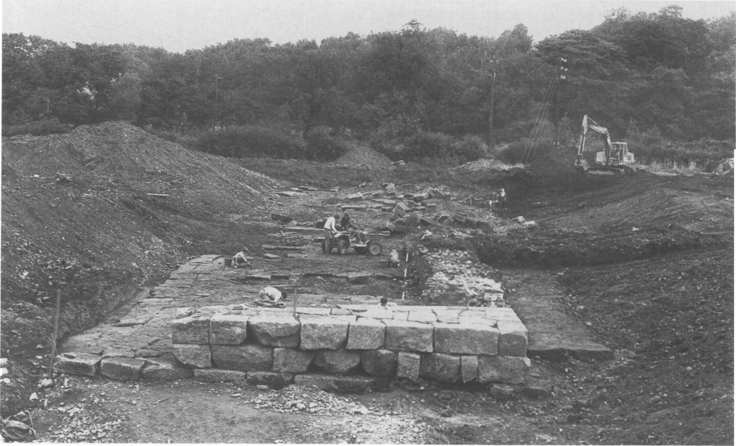
A. Piercebridge: the back of the bridge abutment and pavement viewed from the south shortly after discovery. The robber-trench for Pier 1 is clearly visible in the pavement while to the right of it is part of the later causeway, retained during excavation as a baulk. (p. 118)
