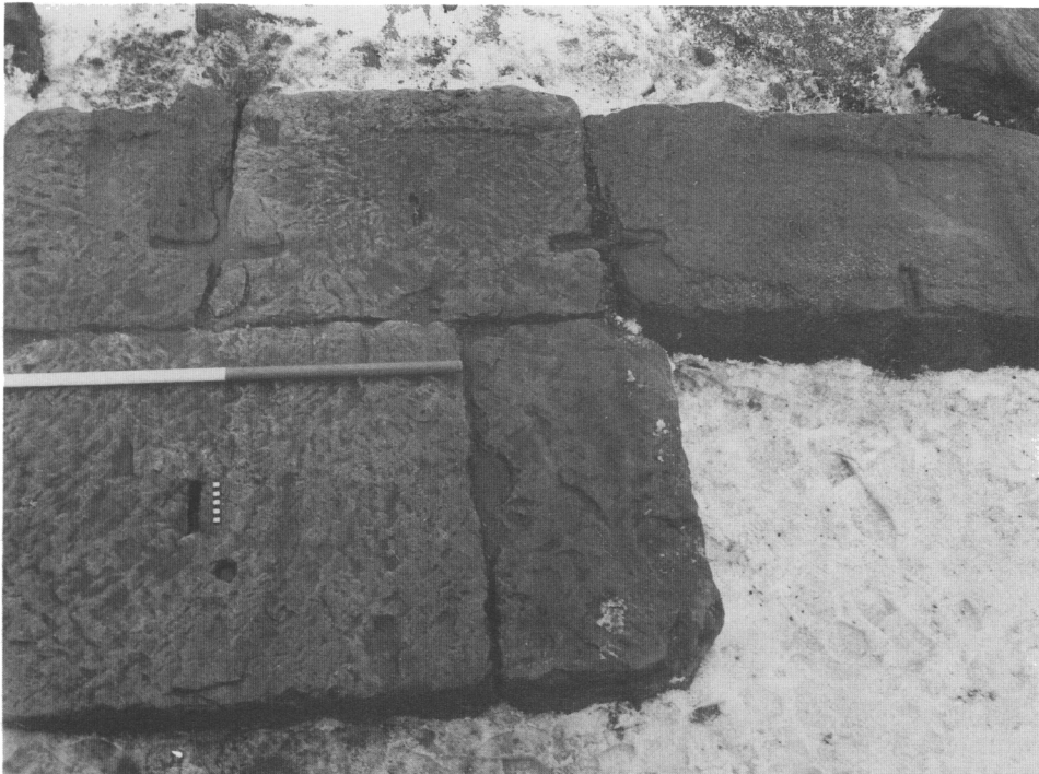
B. Piercebridge: detail of the base of Pier 4. On the right-hand side can be seen the right-angled return of the downwater end of the pier. The whole base is held laterally by iron clamps set in lead. On the face of the stone in the foreground are lewis- and dowel-holes. Scales 0.1 m and 1 m. (p. 121)
