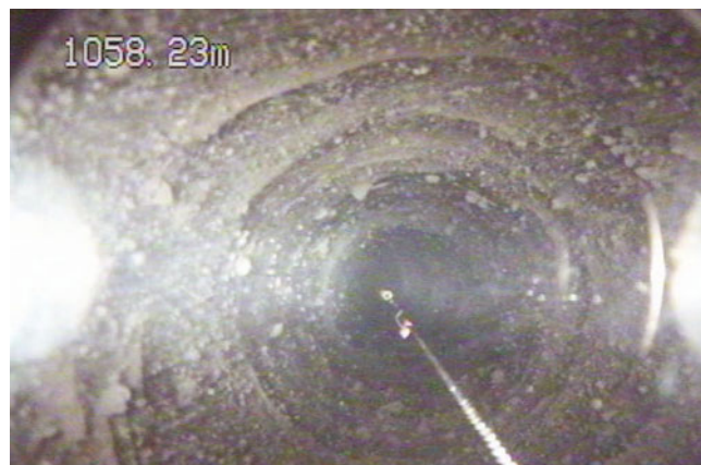
Fig. 14. Elevated debris content, with rocks sticking out from a rough borehole wall.
