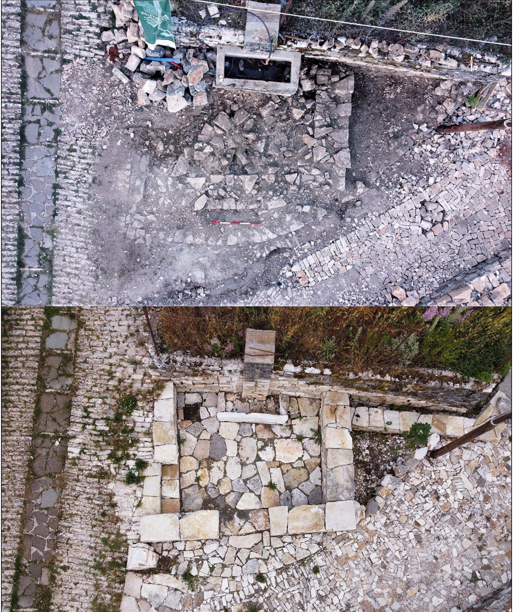
Figure 5. Photographs of the foundations before (above) and after (below) restoration as a public space (photographs by Faidon Moudopoulos-Athanasίου).
