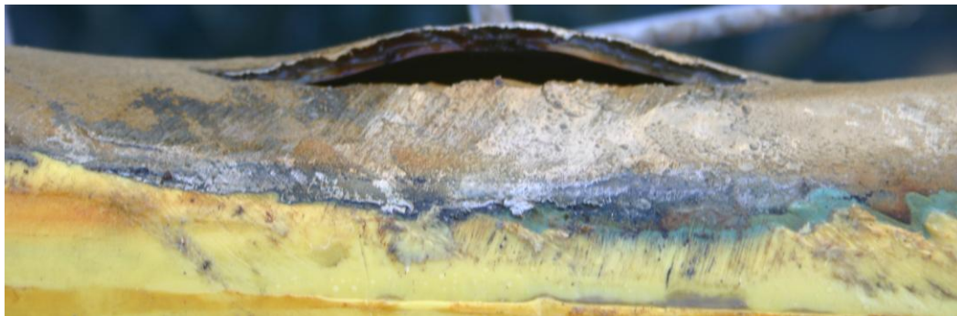
Figure 2: Side view of the cracked methanol pipe (crack is ~4” long) after the surface was ground with a 4” diameter Weiler Power brush during the robot’s initial examination in December 2004.
