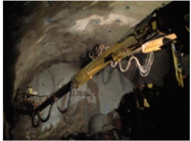
Fig. B1. The drilling machine in use at a tunnel construction site.
