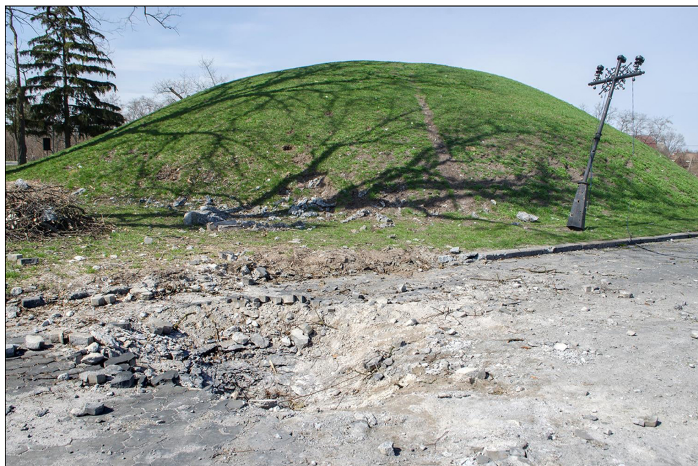
Figure 4. The Princely Barrow dating to the tenth–eleventh centuries AD, located in the north-west area of Boldnyi Hory cemetery, Chernihiv Oblast, Ukraine, was damaged by a Russian rocket strike in March 2022 (figure by Serhii Tarabarov, 2022).
