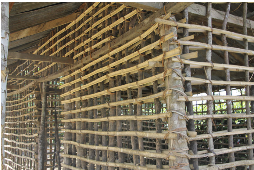
Figure 5. Idu-Èkpèyè village. A family unit dwelling in construction showing structural wall lattice before plastering with wet sand. Change is shown in the installation of a zinc roof instead of thatch. Photo by the author, 2017.
