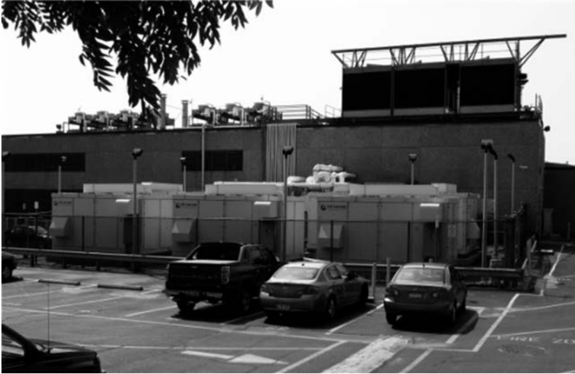
Figure 2.30 Seven fuel cells outside Verizon's Garden City central office.
