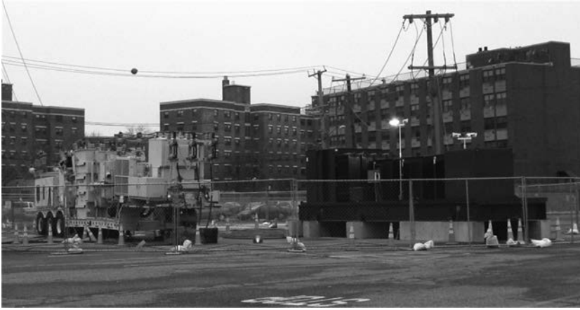
Figure 2.27 Mobile transformer and portable voltage regulators in the parking lot of the Peninsula Family Health Center in Far Rockaway, New York, after Superstorm Sandy.
