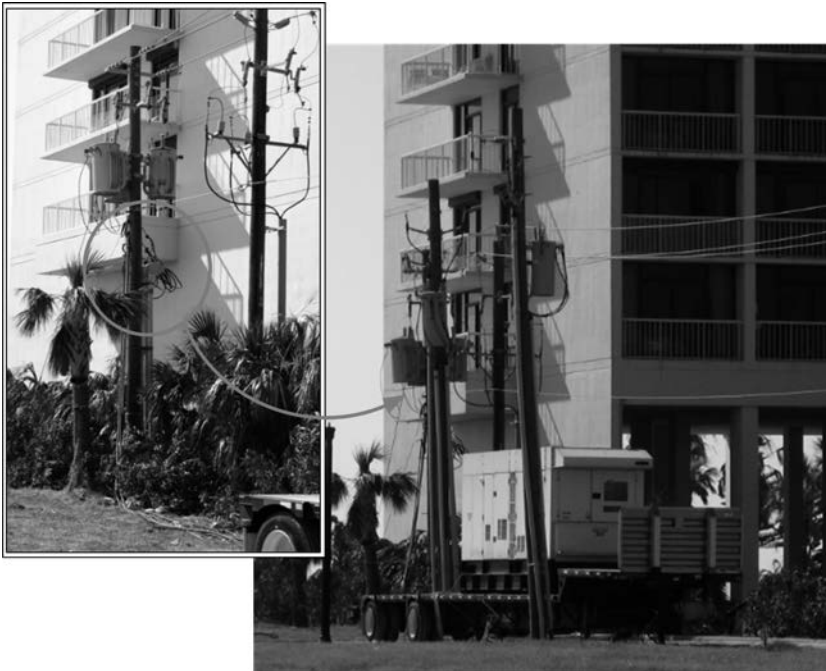
Figure 2.28 A portable diesel genset connected on the power grid side of an apartment complex in Galveston, Texas, after Hurricane Ike.
