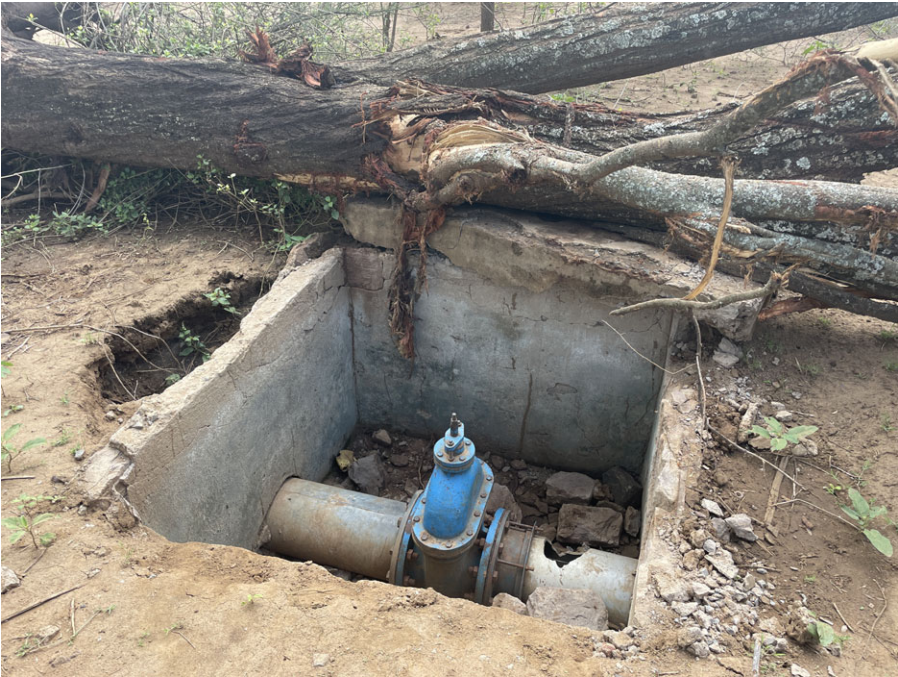
Figure 9. Major damage to piping and pressure valves on the Pokot side of the Tot-Kolowa scheme.
