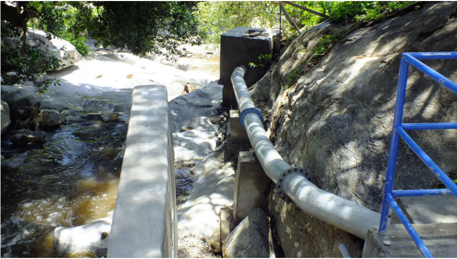
Figure 3a. The main steel pipe exiting the off take.
