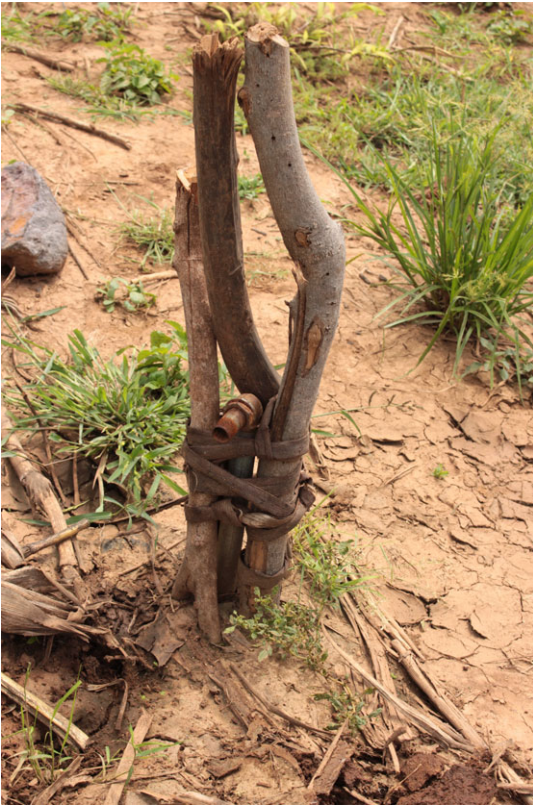
Figure 8b. Ad hoc repairs to a stand-pipe damaged by cattle grazing on the Pokot side in November 2014.
