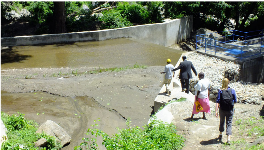
Figure 3b. Concrete off take dam on the Embobut River. Note the extensive silting at the intake already in April 2013.
